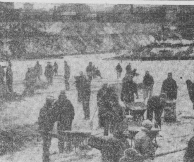
In Cleveland, 1,500 C.W.A. workers have been put to work at this site for a new airport on Cleveland's lake front, which is within a mile of downtown Cleveland. $250,000 of C.W.A. funds are being spent on the airport work.
